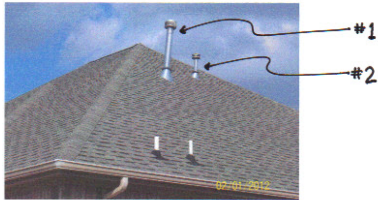
#1 Furnace gas flue and #2 Water heater gas flue
