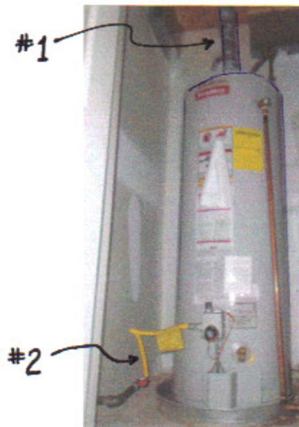
#1 Gas flue #2 Gas line
