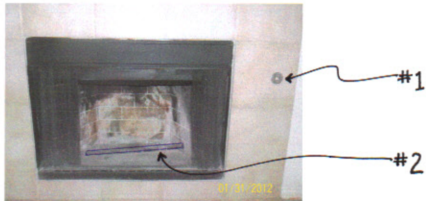
#1 Gas Valve #2 Gas Pipe
