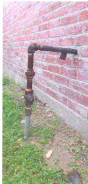
House shut-off valve
